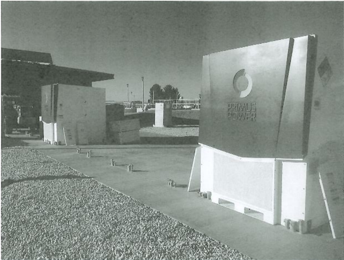
Figure 12: Two Flow Battery Test Units
