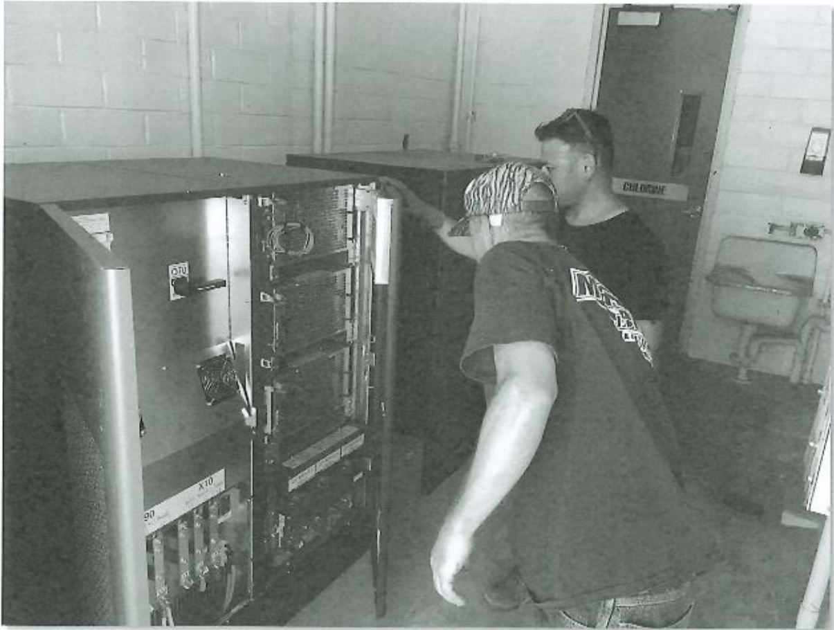
Two Socomec inverters installed indoors.
