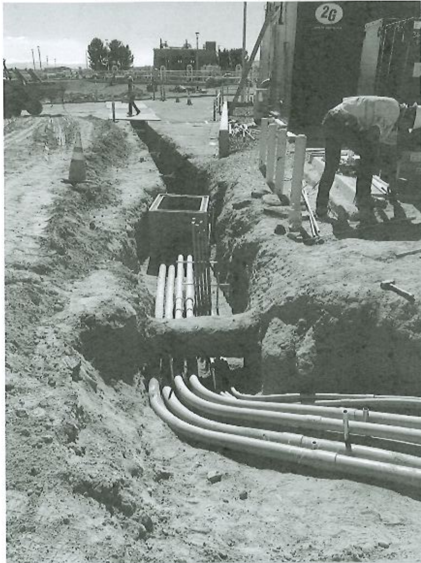
Conduit for power and controls to distribution Panel.
