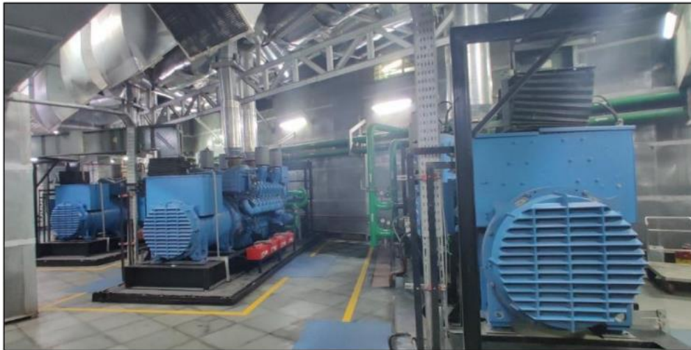
Pic no -32 – DG Sets
