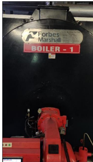
Pic no 24 -Boiler installed in facility
