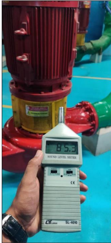
Pic no 6 – Chilled water pump -Sound levels measurement
