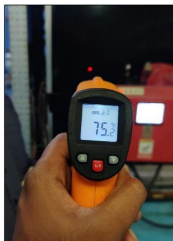
Pic no 25- Surface Temperature – Varying from 61°C to 85°C
