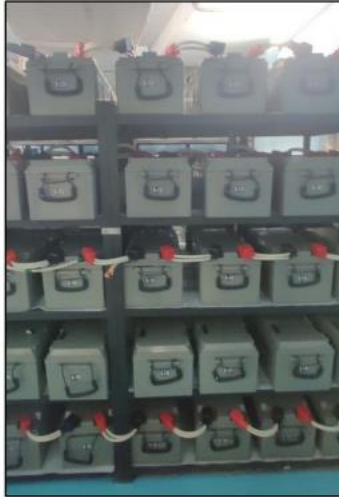
Pic no 31- Batteries
