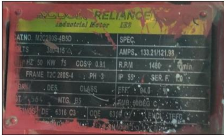
Pic no – 10 - Motor specification tag
