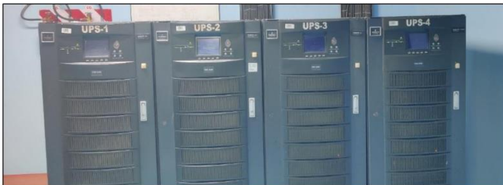
Pic no -30 - UPS
