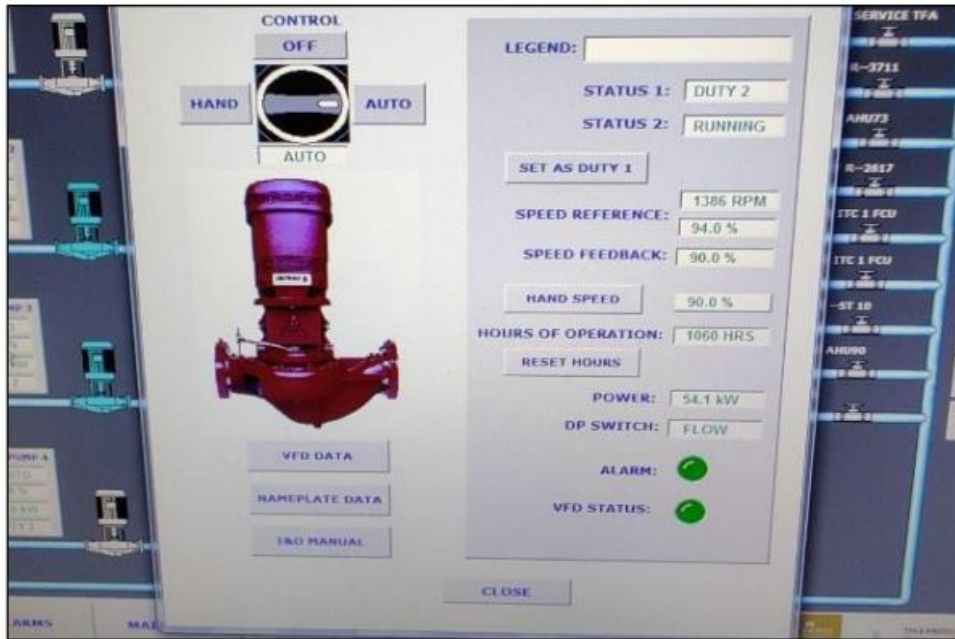
Pic no 9 - Chiller pumps parameters in Building management system
