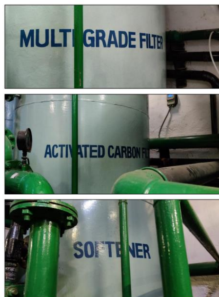
Pic no 36- Water Treatment plant
