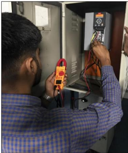
Pic no 12-Field Electrical load measurements
