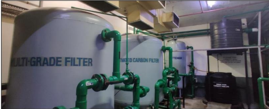
Pic no 37 - Sewage & Effluent Treatment Plant (STP & ETP)
